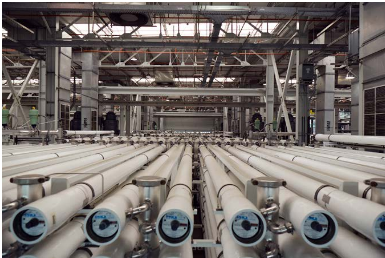
Reverse osmosis units at the Orange County Water District's Groundwater Replenishment System plant. (photo credit: Orange County Water District).
